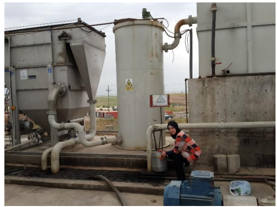
Figure 2. The untreated wastewater
